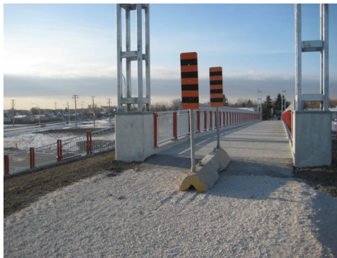
Northeast Pioneers Greenway bicycle/pedestrian bridge over Chief Peguis Trail- photos by Kevin Miller
