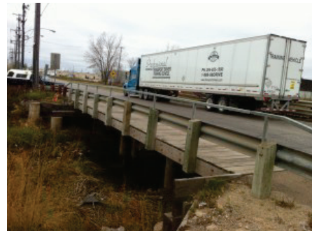
Saskatchewan Avenue Omand's Creek Bridge – Schedule for reconstruction in 2016, it should be possible to provide a good quality connection between protected bike lanes on Midland Street and those planned for Empress Street, as well as to the off road pathway planned for the north side of Saskatchewan Avenue west of Empress Street.
